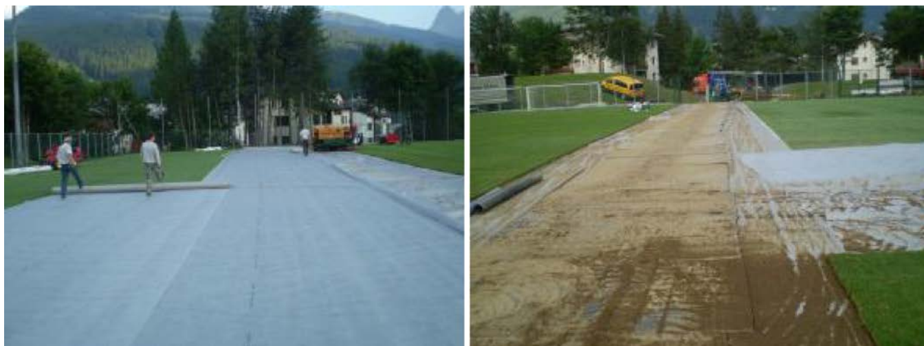
Installation of DuPont™ Typar® on the ground of Bardonecchia's football field; photos by Bruno Marabotto, all rights reserved.
