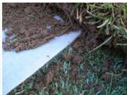
detail of the ground with DuPont™ Typar® geosynthetic applied 施工グラウンド、近接
