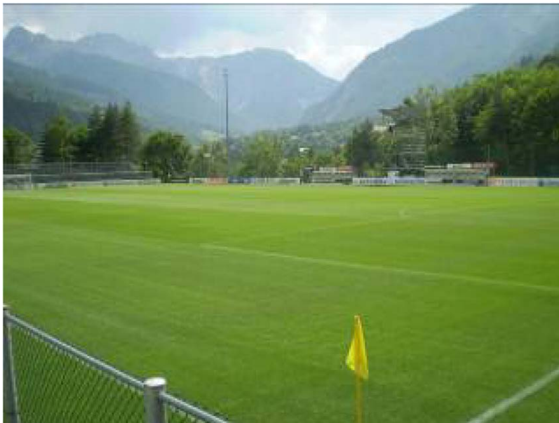
Bardonecchia football stadium: the new field with natural grass placed on DuPont™ Typar® geosynthetics; photo by Bruno Marabotto, all rights reserved.
